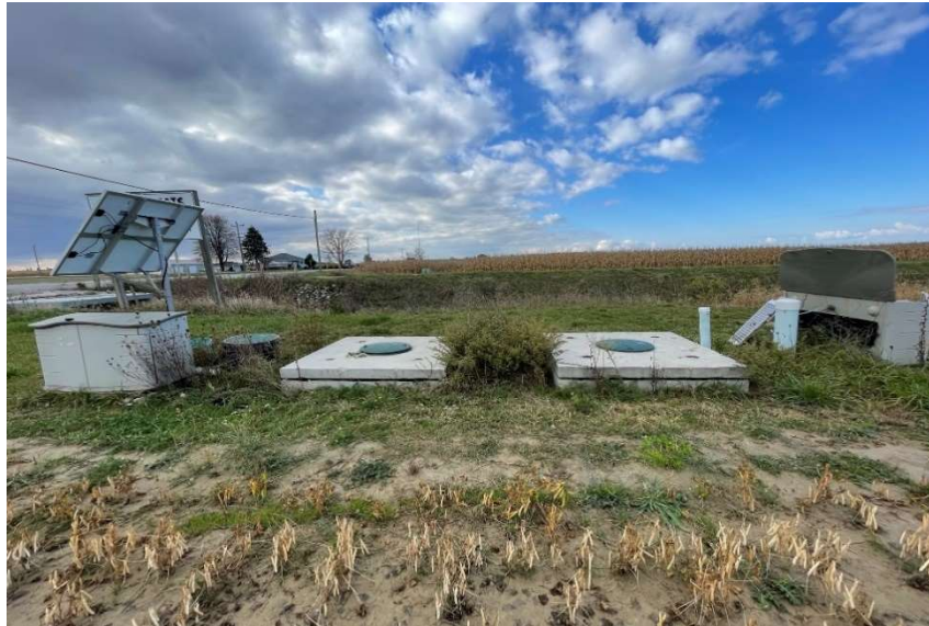
Figure 6. Fairview site containing an inflow permanent ISCO enclosure with solar panel [Right], first tank [Right Middle], second tank [Left Middle], and outflow permanent ISCO enclosure with solar panel [Left].
