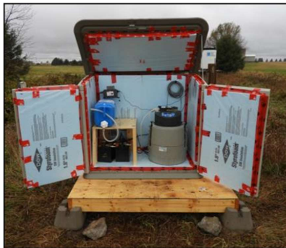
Figure 3. The inside of a water monitoring station established by UTRCA
