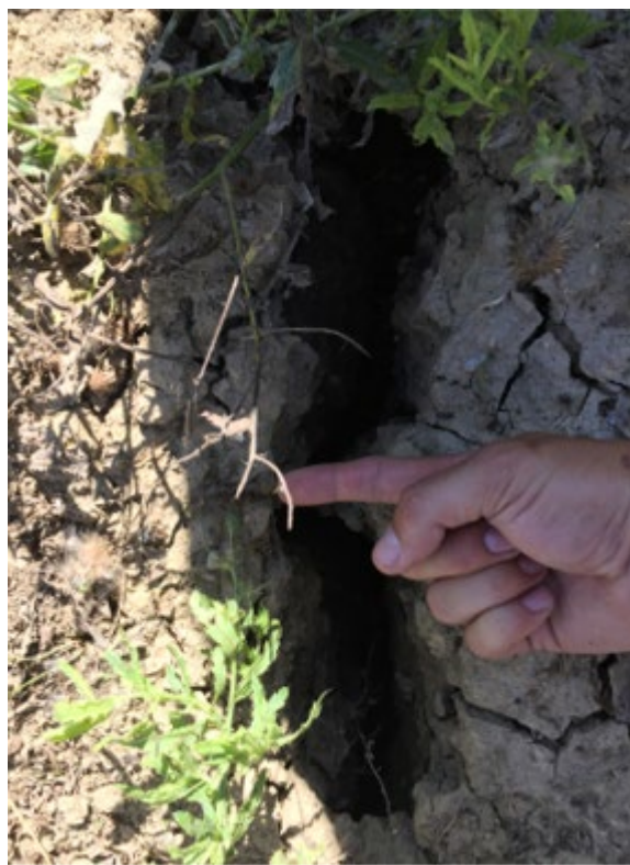
Figure 15. Photograph of a sizeable crack forming in Brookston Clay soil from the Deary Pump Station subwatershed.
