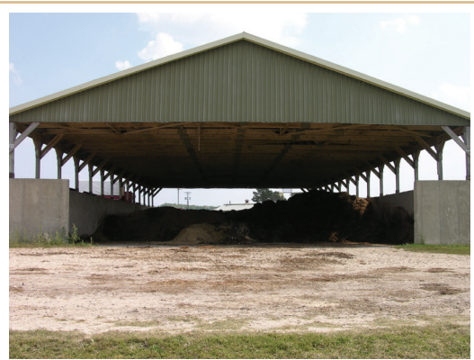
Eliminating direct rain and snowfall will free up available manure storage capacity.
