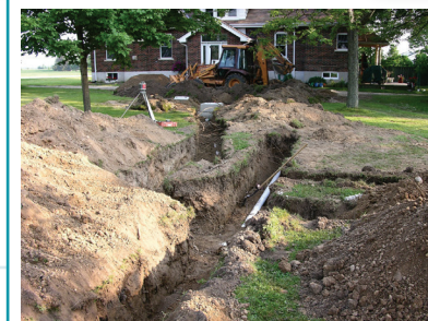
Ensure that the sewage system has a Building Permit or Certificate of Approval and that it was adequately sized and installed by a licensed installer.
