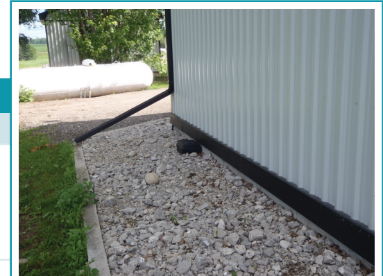
Eave troughs, foundation and footing drains should be separate systems in no way connected to the sewage system.
