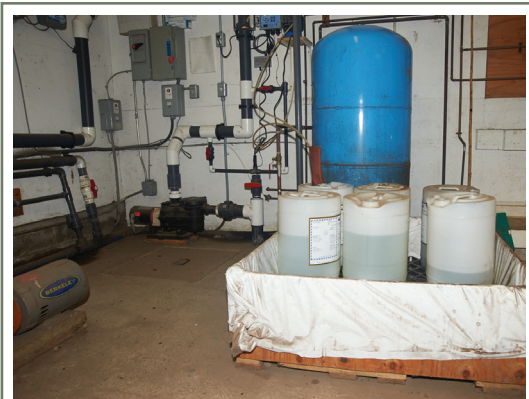
Liquid materials warrant special precautions, such as secondary containment.
