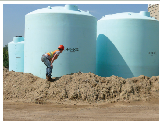
Scheduled monitoring of both the storage and the containment area reduces the risk of loss of material.
