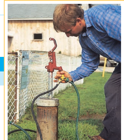
This drilled well metal casing has a frost-free hydrant faucet with an anti-backflow device.
