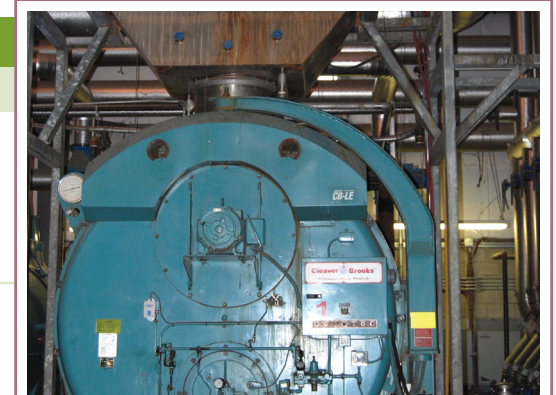
Capturing heat and CO 2 from flue gas allows for the recycling of energy that would otherwise be wasted.
