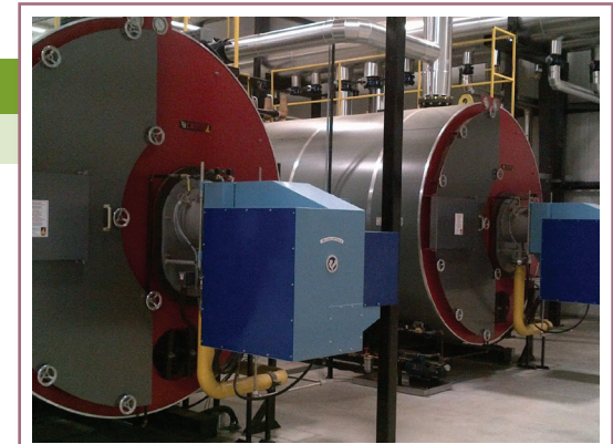
Regular boiler maintenance enhances heating efficiency.
