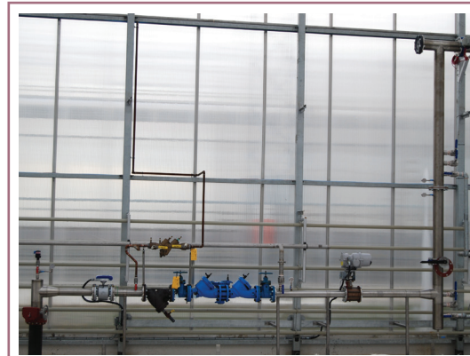
Whenever fertigation equipment is used, always check that anti-backflow devices are installed and operating properly to prevent any backflow contamination of the water system.
