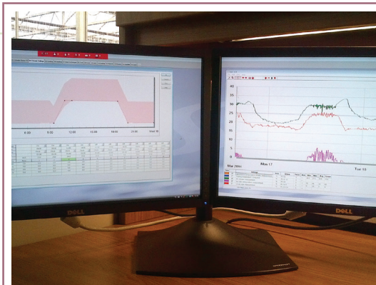
Using computerized controls in greenhouses can mean significant savings in energy consumption and costs.
