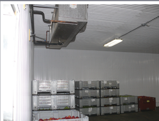
Ensure the refrigerated storage facility is insulated and sealed to prevent the entry or escape of air and provide good air distribution within the storage.
