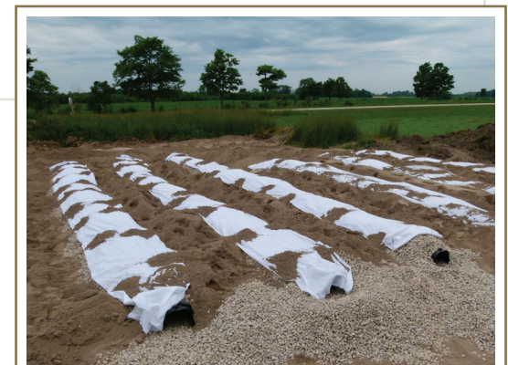
This treatment trench area will be fenced off from livestock and vehicles once installation is complete.
